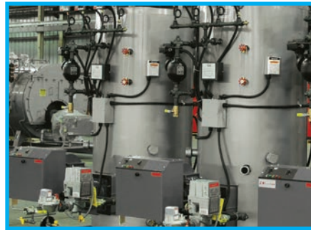
Power Boiler and Heat Exchange Manufacturing NAICS Code 33241
